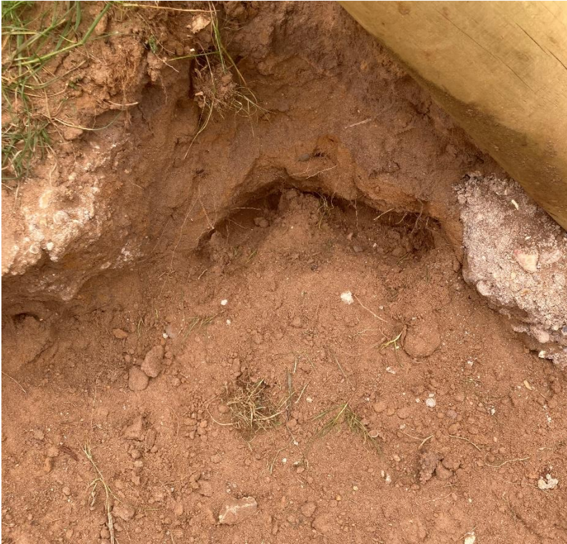
Holes created by sticks used to undermine foundations
